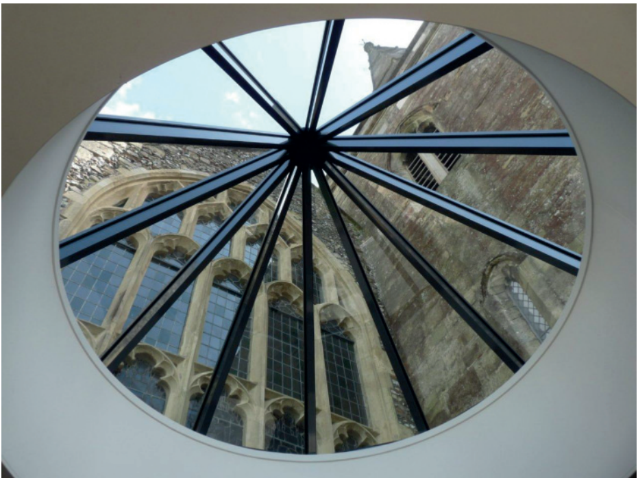
A dodecahedral Lantern was the most striking feature of this major improvement to the entrance and porch to St Martin's Church, given an Award.
